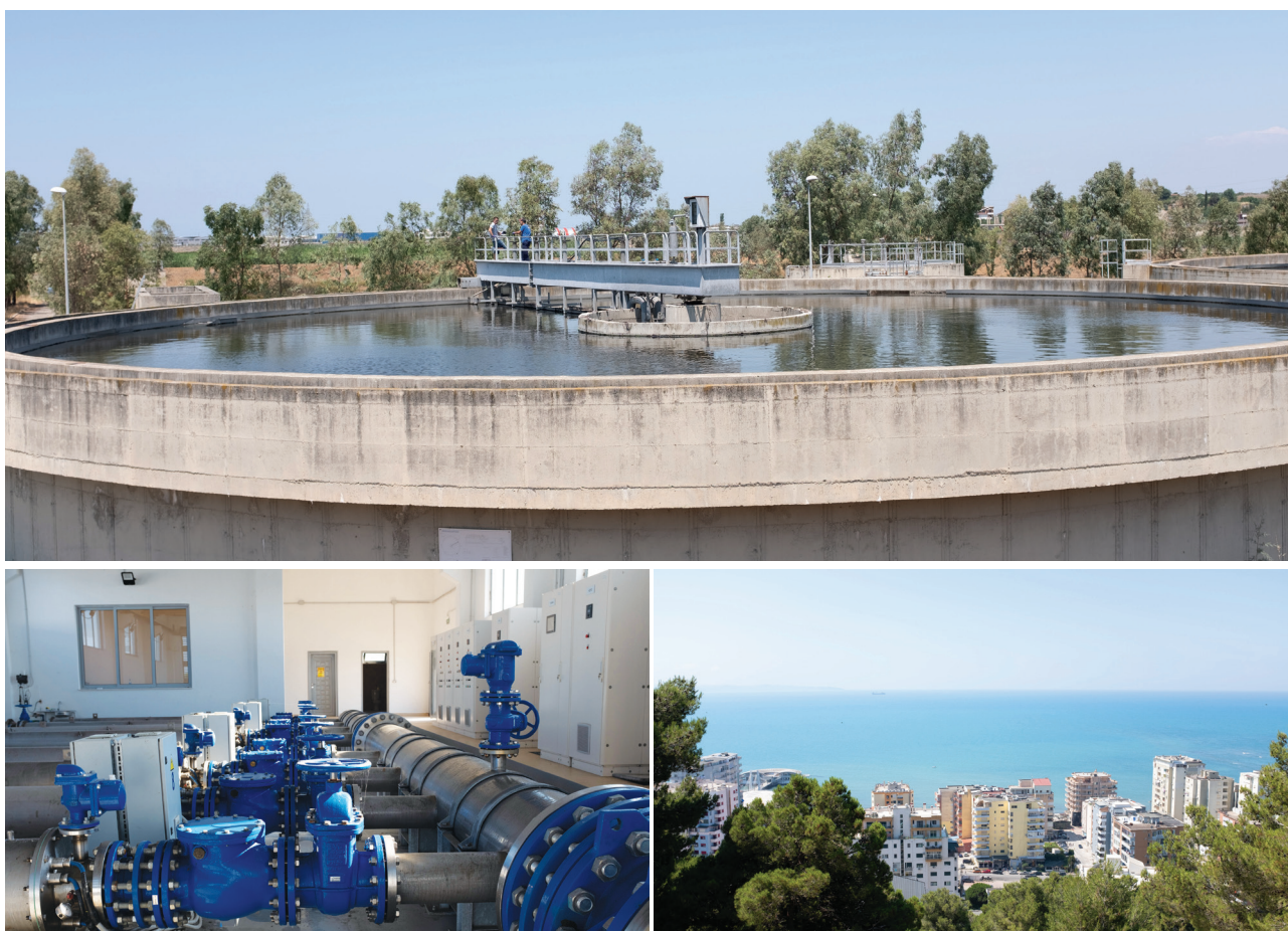
Albania/ Durres Wasterwater treatment plant © Marie Tihon / AFD
